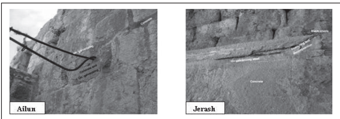
Fig. 3 a, b: Shows deterioration appearances resulting from the effects of using Reinforced Concrete
